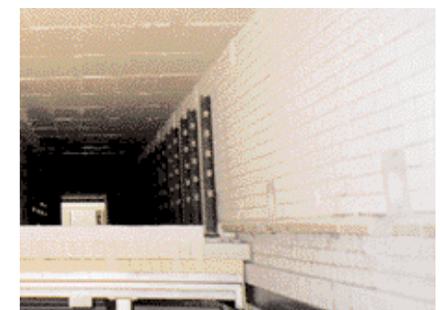
Tunnel kiln for the ceramic industry
