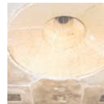
Burner brick in pusher furnace for the steel industrie
