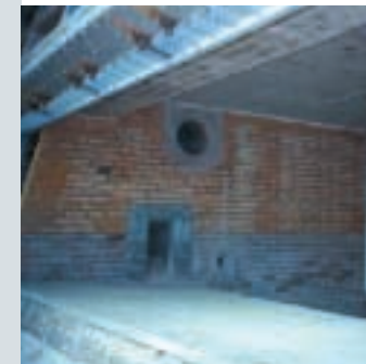
Melting furnace for the aluminium industry
