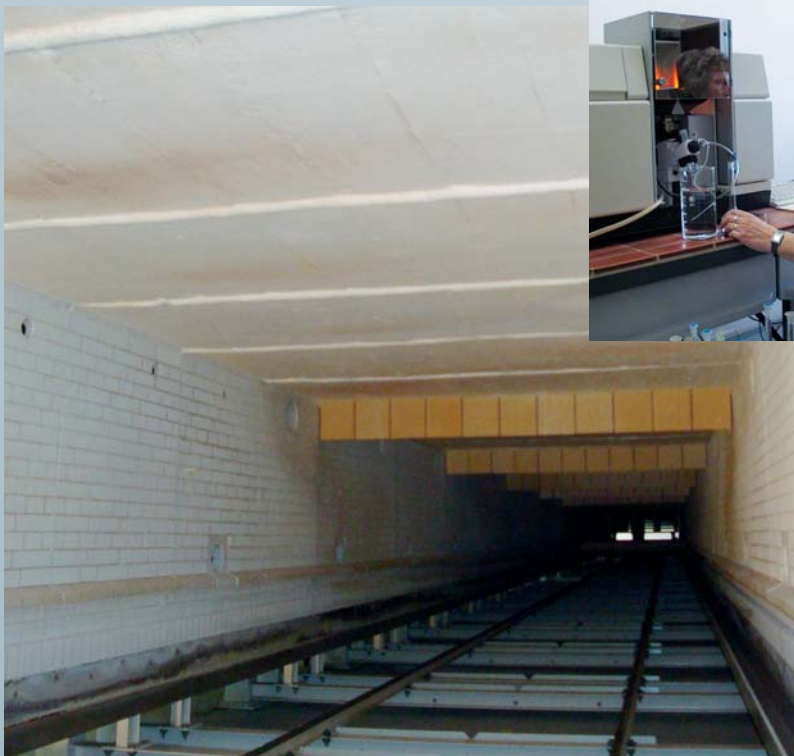
Tunnel furnace sanitary ceramics after 8 years operating time
