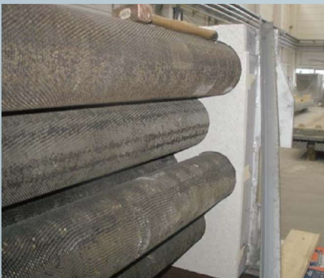
Convection zone tube shield (petrochemical cracker)
