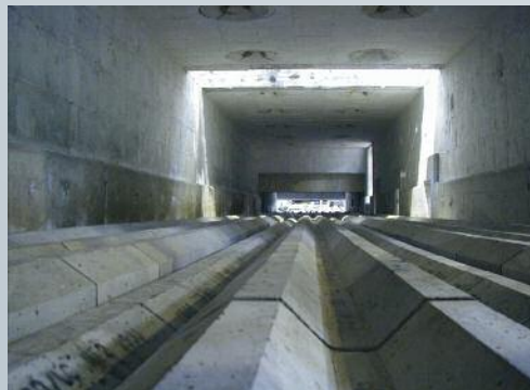
Walking-beam furnace with pre-cast shapes
