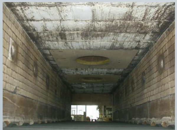
Roller furnace after 5 years of operation
