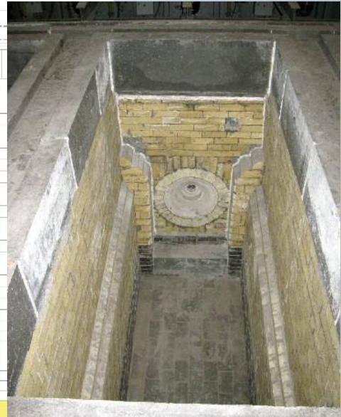
Soaking pit furnace
