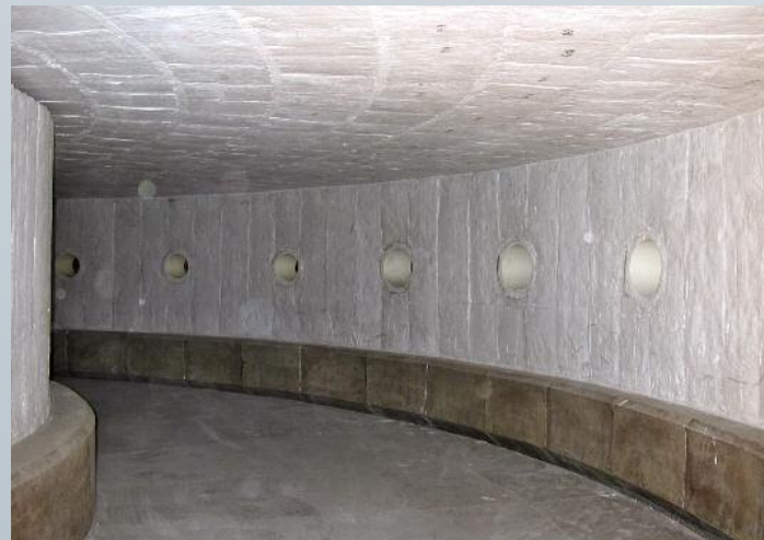
Rotary hearth furnace with module lining
