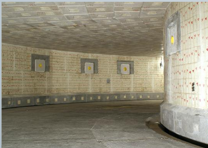
Rotary hearth furnace with dense lining
