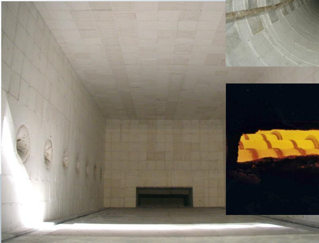
Bogie hearth furnace with module lining
