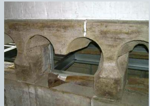
Castable lining in roller furnace
