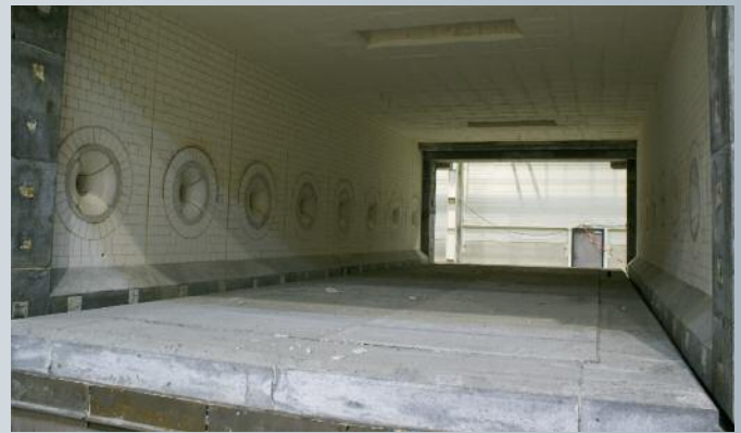
Forging furnace with insulating brick walls and module ceiling
