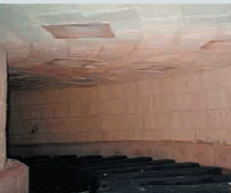
Rotary hearth furnace
