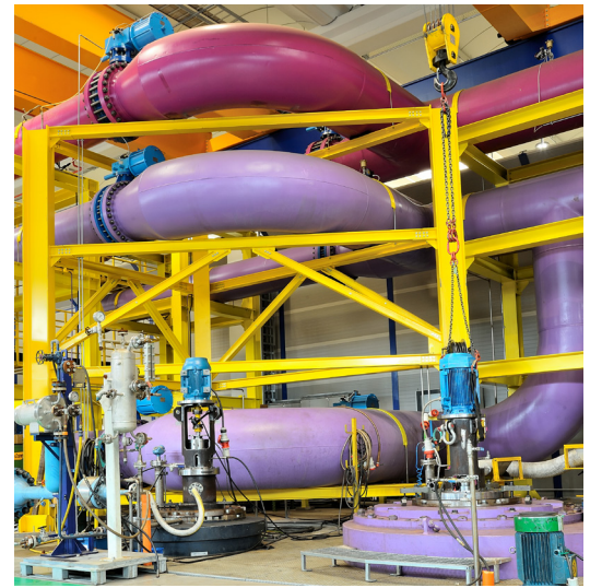
Vertical pump benches
